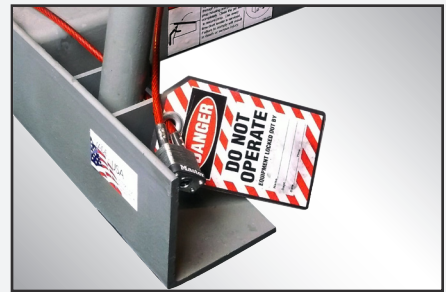
Lockout/tagout maintenance strut and lip supporting service strut.
